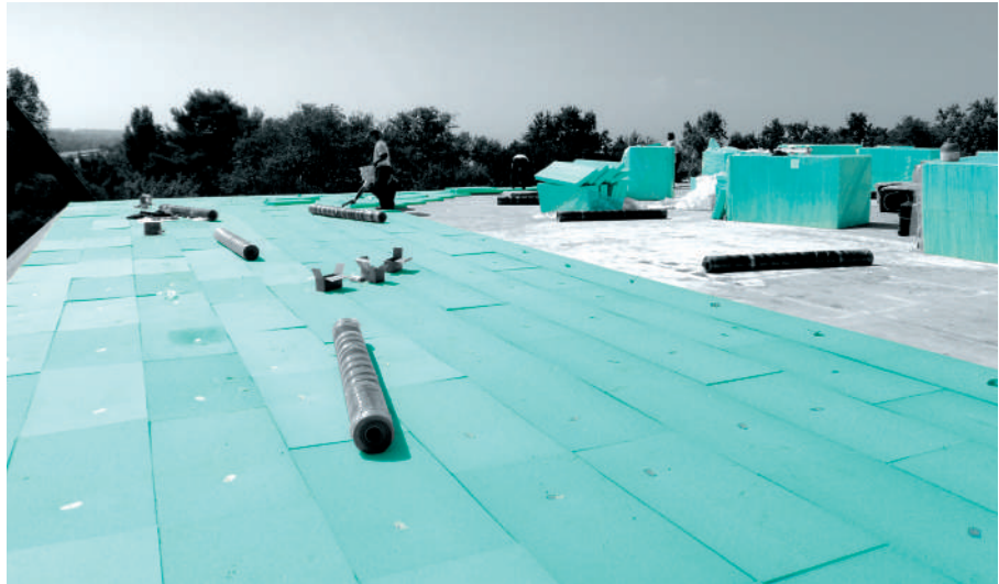
Increasing the roof slope by using FIBRANxps INCLINE and simultaneous flat roof thermal rehabilitation.
