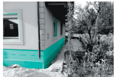
Resolving thermal bridges on window and door jambs and thermal insulation of façade plinths with FIBRANxps ETICS .
