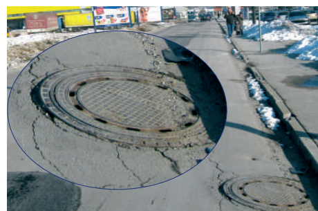
Freezing of marshy ground, soaked with water, causes damage on roads and sewage systems.
