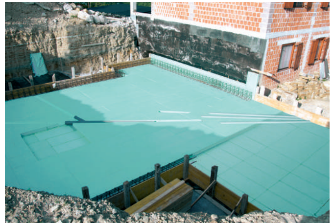
Installation of services into previously cut out channels of FIBRANxps thermal insulation boards.
