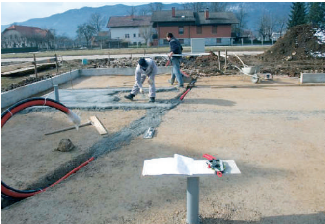
Vertical service installation, compacting and levelling out of the ground, on which the first layer of FIBRANxps 400 - L insulation will be placed.
