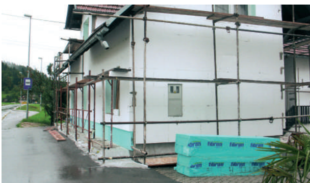
The execution of thermal insulation of facade plinth is described in detail in leaflet No. 0130 – Facades – Building instructions.
