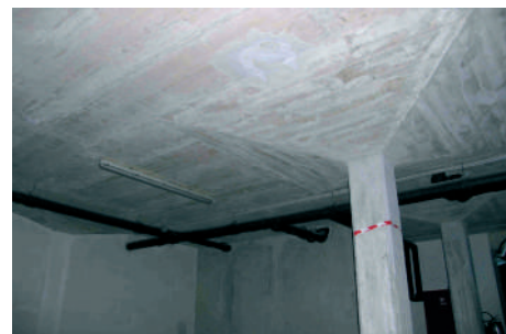
Consequence: huge energy loss and non-comfortable living. In heated spaces above the cold basement condensate and mould are visible.
