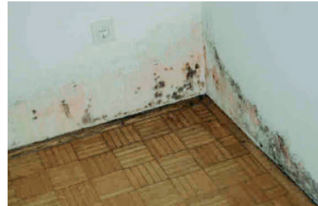
Visible moisture and health damaging mould on the wall.
