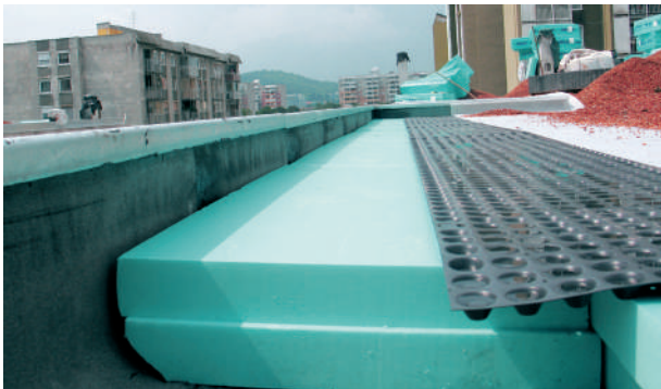
The execution of thermal protection of green roofs is described in detail in leaflet No. 0111 – Inverted flat roofs – Building instructions.
