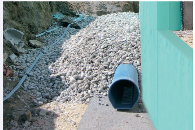
To ensure the optimum performance of thermal insulation, it is advisable to install an adequate drainage system around the entire thermally insulated object, to allow drainage of rainwater and underground water.
